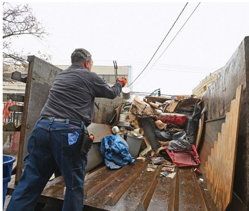
GNJ volunteer loads debris into dumpster during clean up in Jersey City
